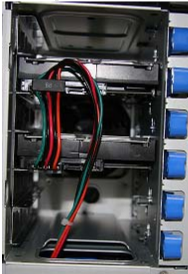
Current cable assembly
